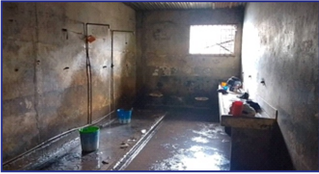
A bathroom in one of the cells in the Port Loko CC
